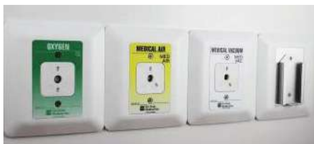
Recessed Ohio Outlets
